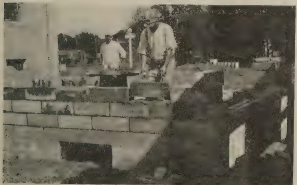
Stone masons in the employ of the Concrete Stone Company, Davenport, Iowa, set a record hard to beat—laying over 400 concrete blocks each day
